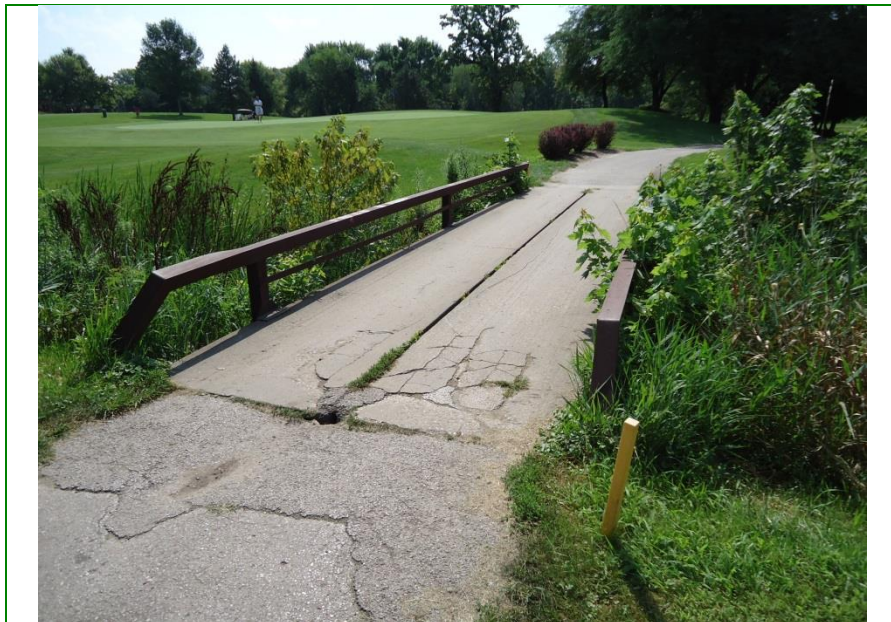
One example of the condition of the bridges at Palmer Hills GC that will need to be repaired or replaced within the next five (5) years.
